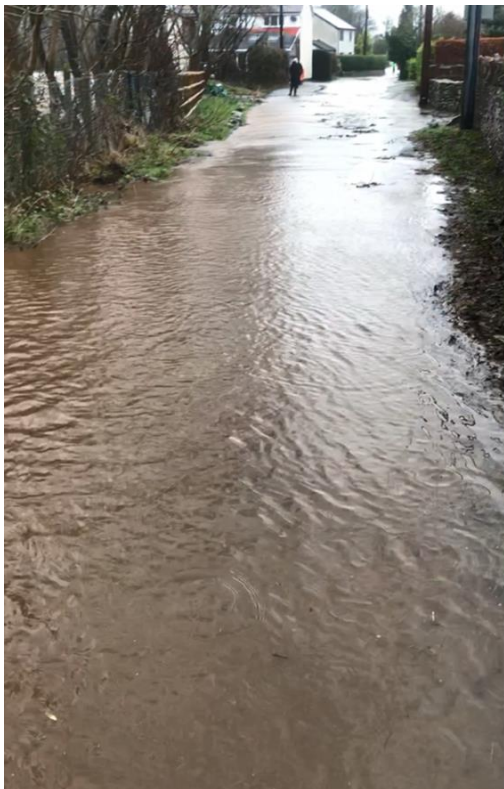
Figure 7: Overtopping between Plas Estyn and Quillet. Source: Resident
