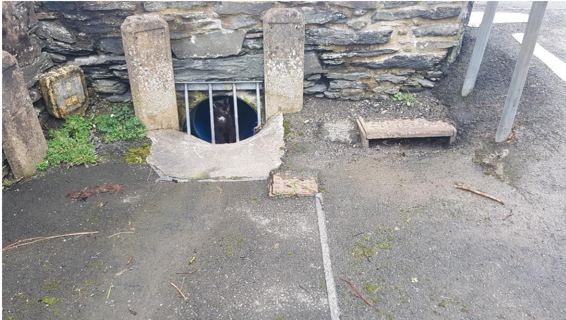
Figure 10: Flood relief culvert at the High Street road bridge. Source: NRW staff
