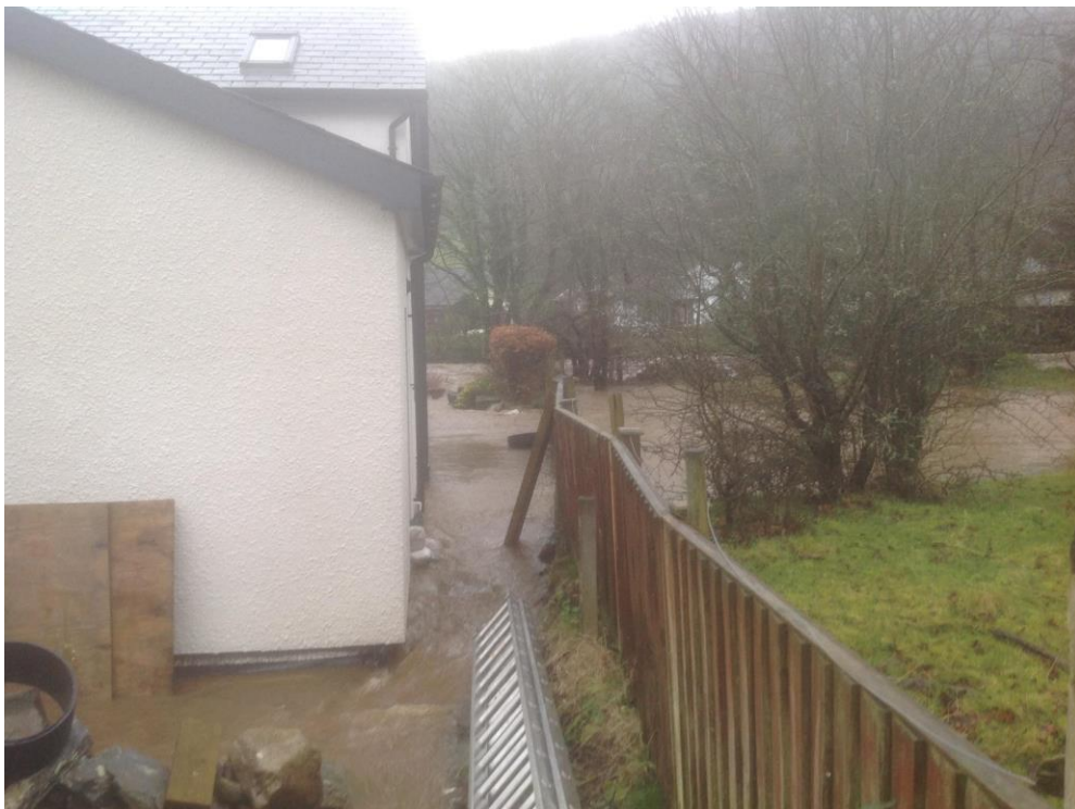
Figure 12: Floodwater at the rear (south) of Glan Ceidiog. Source: Llandrillo Facebook group
